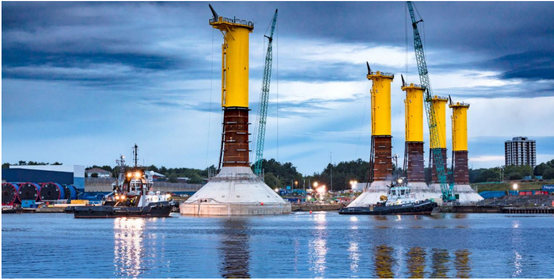
Figure 4.20 Blyth Offshore Demonstrator project – using floating GBS constructed in a dry dock
